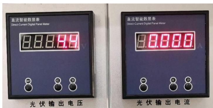
Figure 1 DC Voltmeter and Ammeter
